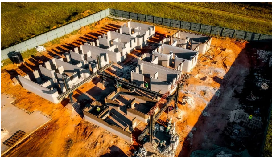
Aerial view of the construction site: 3D-printing enables fast, resource-efficient and cost-effective construction.
