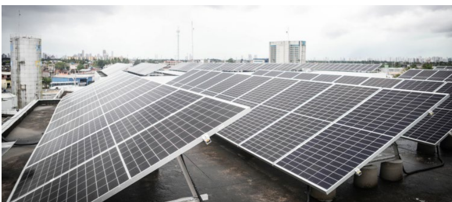
Photovoltaic solar plant at the Dr. Mercês Pontes Cunha Women’s Hospital in Recife (HMR) ©Rodolfo Loepert, PCR
